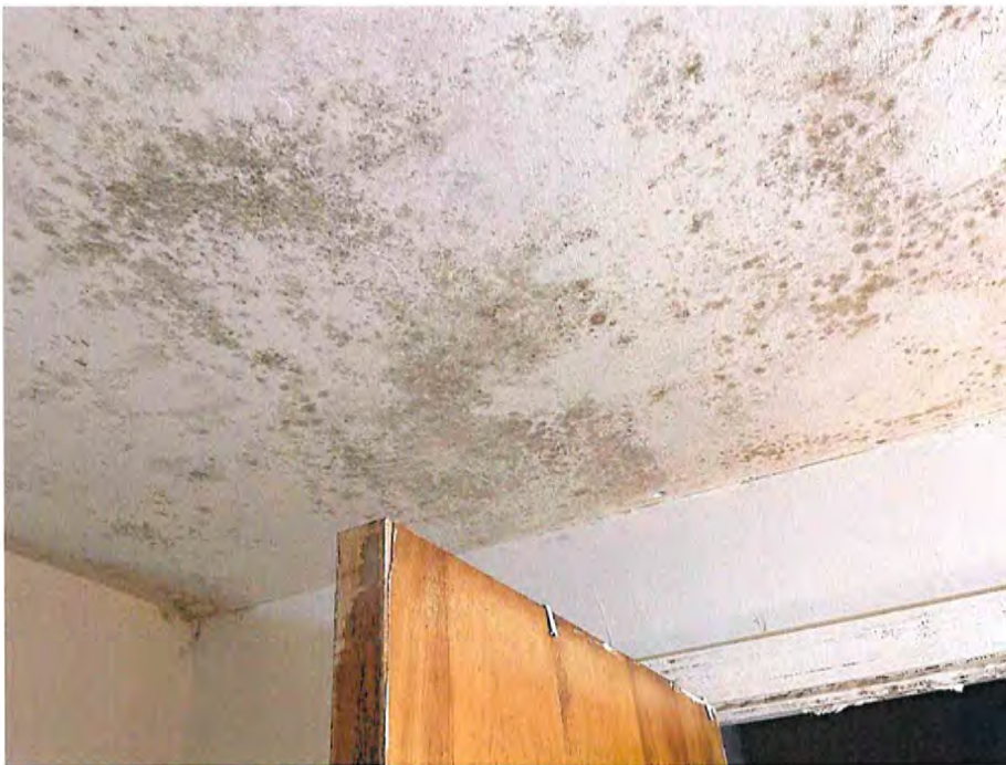
Photo-6 Plaster ceiling 2 nd floor bathroom.
