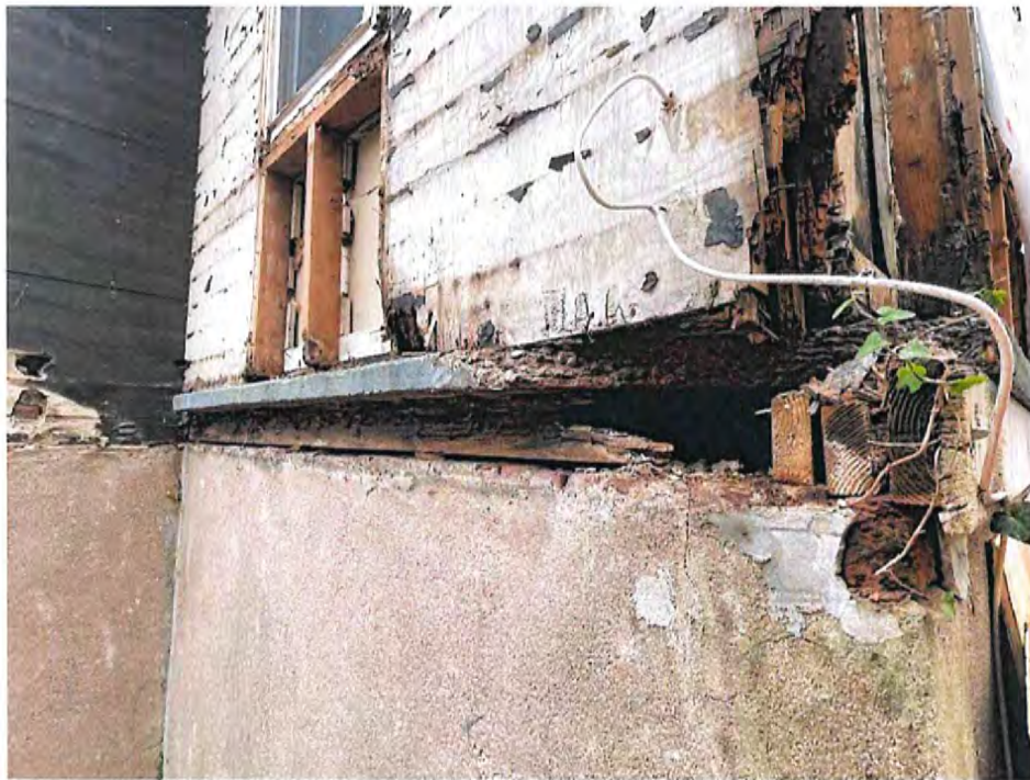
Photo 4- Damaged wood sill and concrete floor slab
