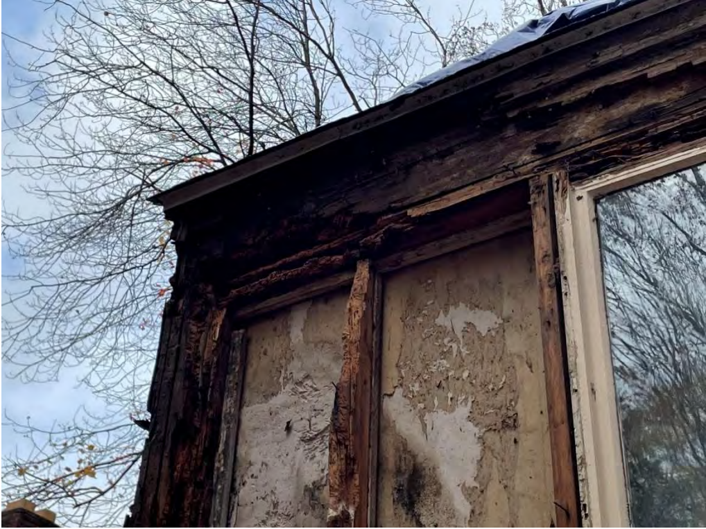
Photo 3- Damaged wood header
