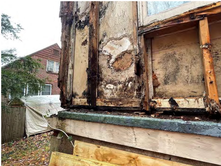
Photo 2- Damaged wood Framing
