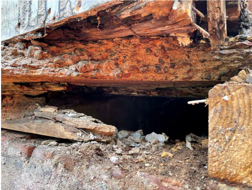
Photo 5- Damaged wood sill and concrete floor slab (close-up)
