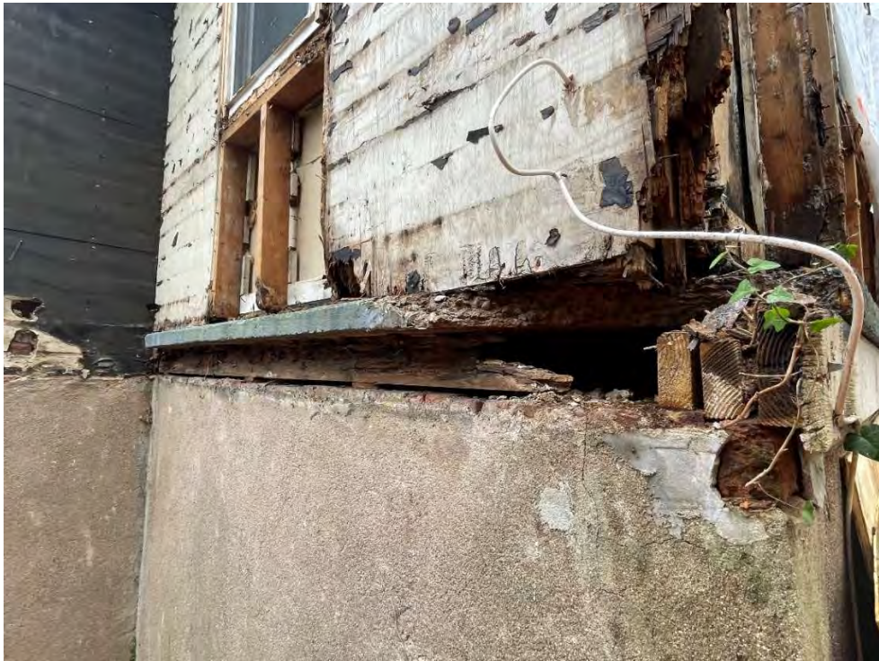
Photo 4- Damaged wood sill and concrete floor slab
