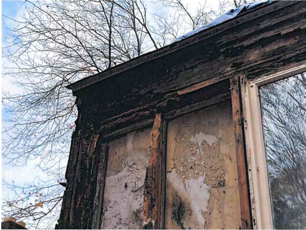
Photo 3- Damaged wood header
