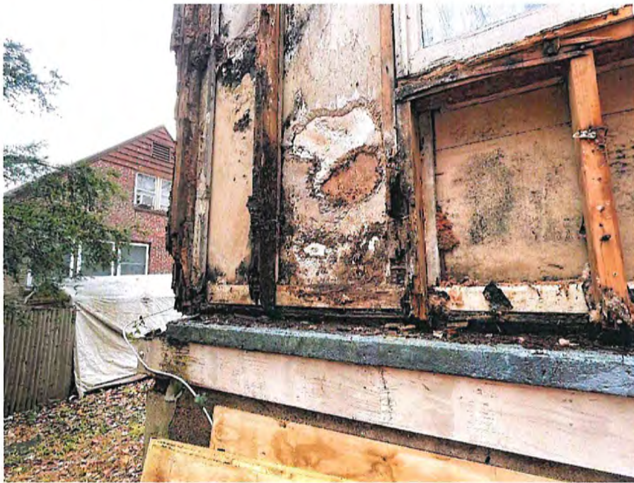
Photo 2- Damaged wood Framing
