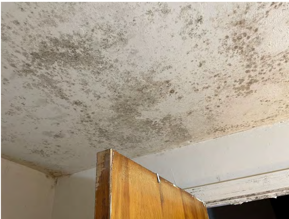
Photo-6 Plaster ceiling 2 nd floor bathroom.
